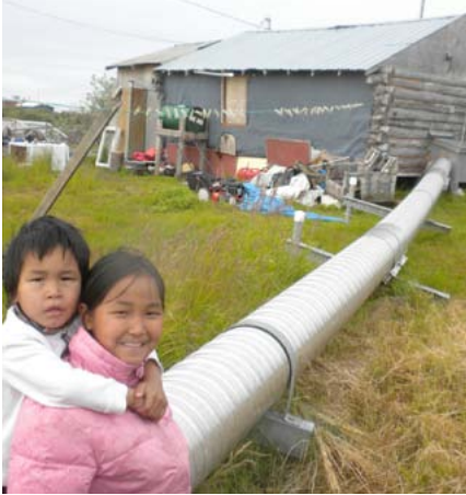
Children playing near sagging waterline in Selawik, Alaska.
